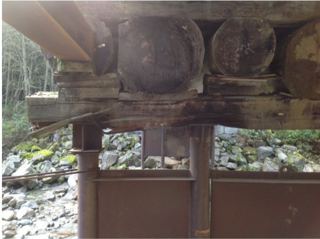
old structure timber cap crushing
