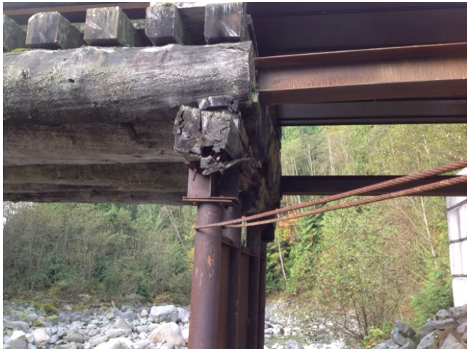
old structure timber cap rotten and crushing
